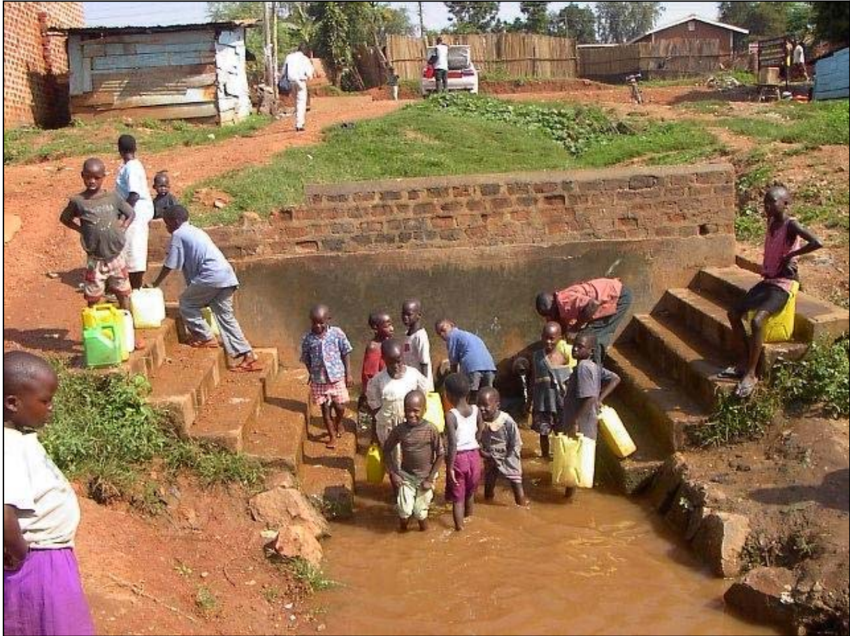
Fig. 30 Protected spring within the study area. Note the damaged spring protection wall and loss of cut-off drain, which contribute to direct entry of surface contaminants into the spring backfill during the rains
