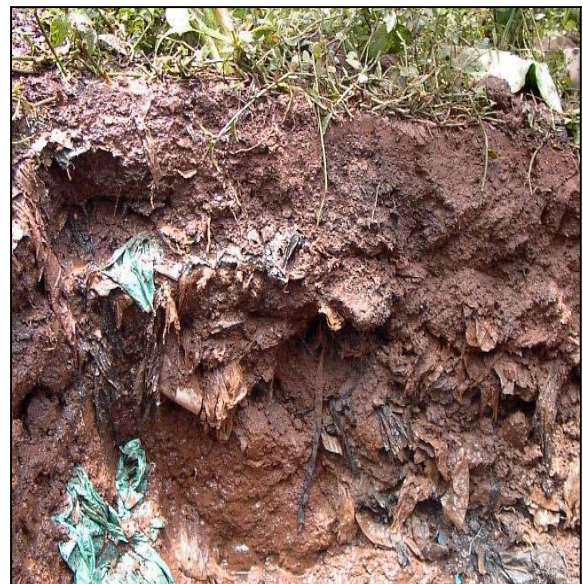
Fig. 29 Trial pit at MW 15 location exposing the profile. Note the presence of foreign material which bring about macropore flow
