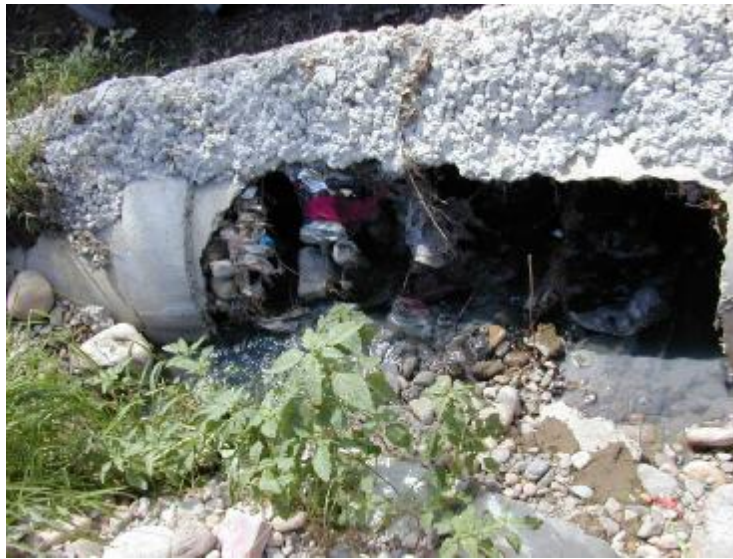
Uncontrolled wastewater discharge at new sewer
