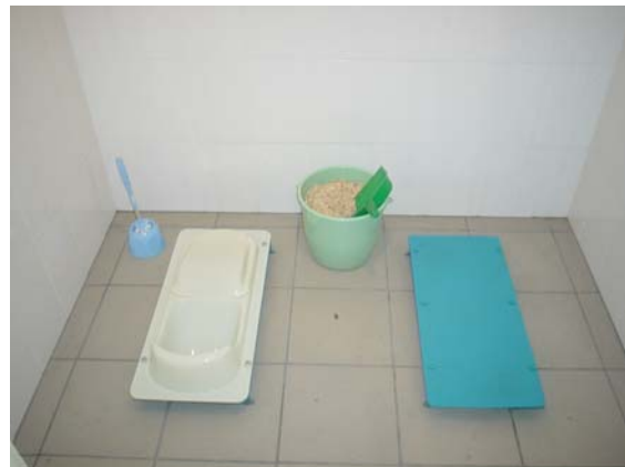
Figure 4. Urine diverting squatting dry toilet from Ukraine
