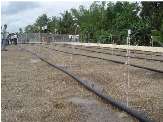
Fig. 7: Testing distribution system of wastewater on vertical soil filter (cell 1 of constructed wetland), June 2006 (source: DILG-GTZ Program).
