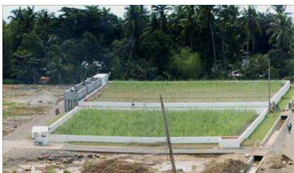
Fig. 8: Constructed wetland when construction was just completed in September 2006 (source: GEOPLAN Cebu).
