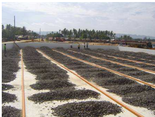
Fig. 5: Preparation of drainage system of cell 1 of the constructed wetland (vertical flow), January 2006 (source: DILG-GTZ Program).
