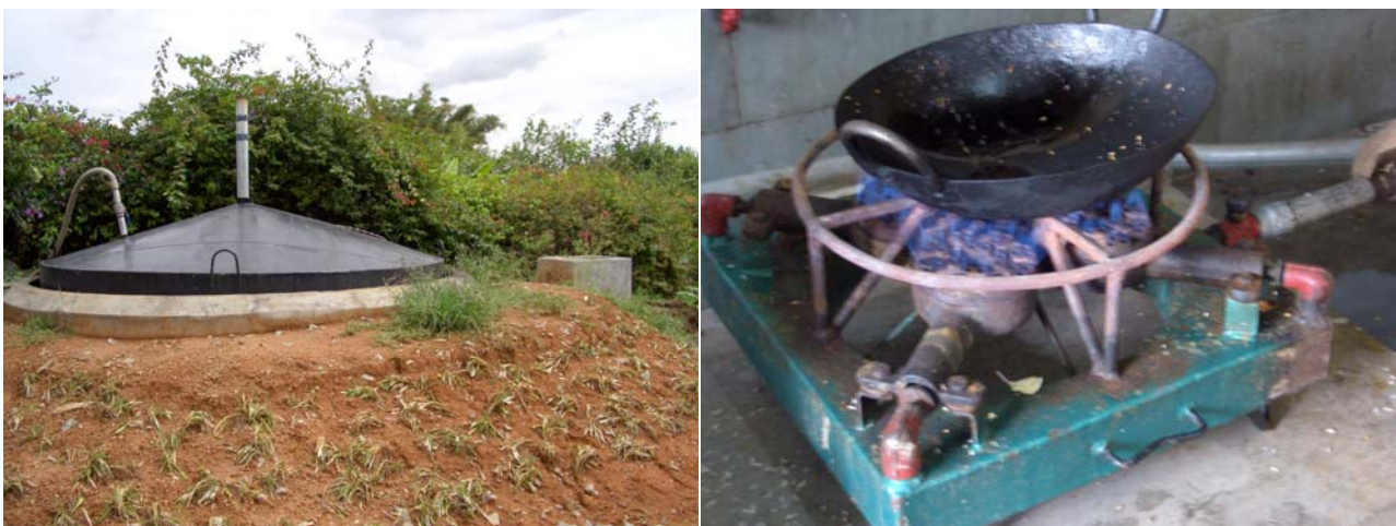
figure 3: New biogas plant at ACTS Rayasandra Campus (left) and use of biogas for cooking (right)
