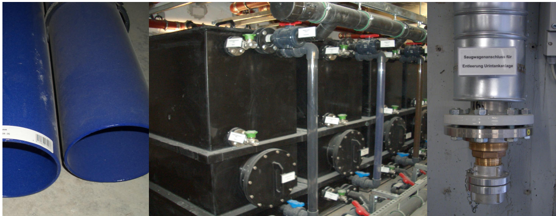
Figure 4 Pipes of cast iron with enamel coating (left), urine tanks (middle), and docking station for tank trucks (right) (source: GTZ)
