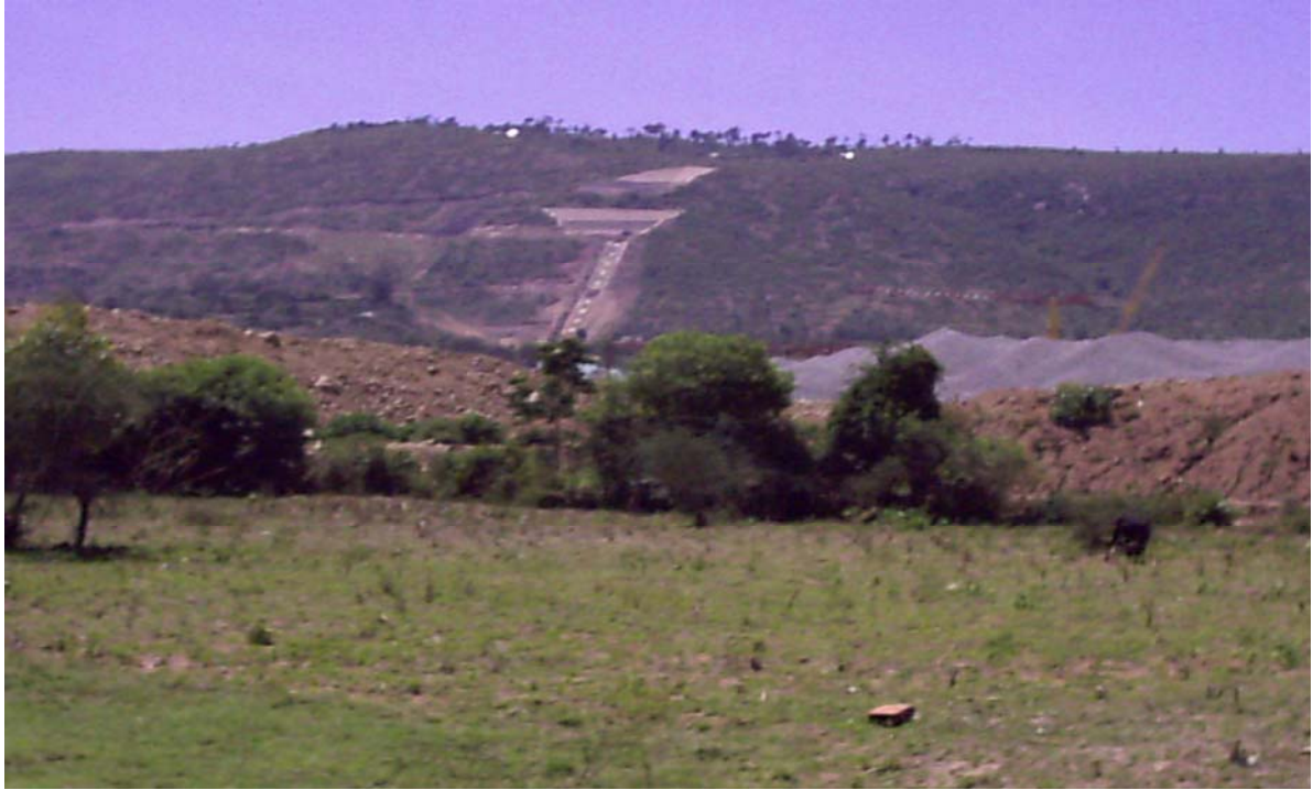
Sondu Miriu project: Far background - Headrace channel on Nyakach escarpment to power house Middle ground - Excavated material stocks and crushed Ballast Next to powerhouse
