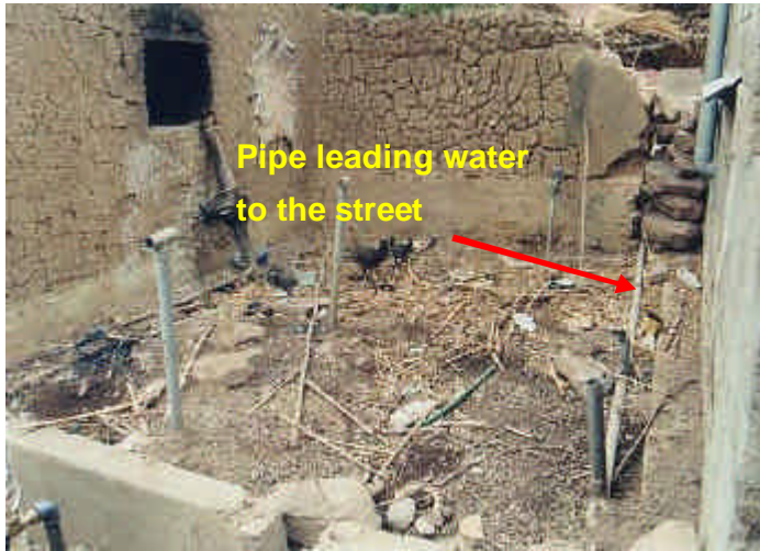
Figure 2-11: Photo of wastewater garden
