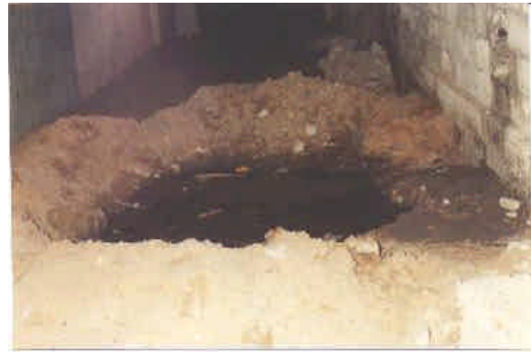
Figure 1-6: Sewage hole in the road
