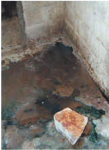
Figure 3-8: Extensive concrete corrosion
