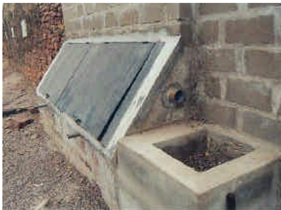
Figure 2-21: Metall cleanout access door and drainage effluent chamber
