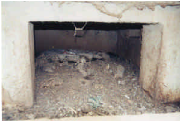
Figure 2-14: Unused dessication chamber filled with faeces
