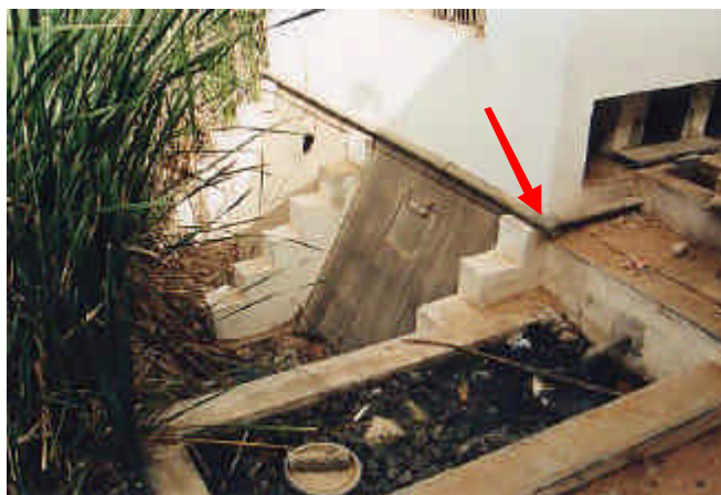
Figure 3-3: First basin and metal cleanout acces door of the ecosan system
