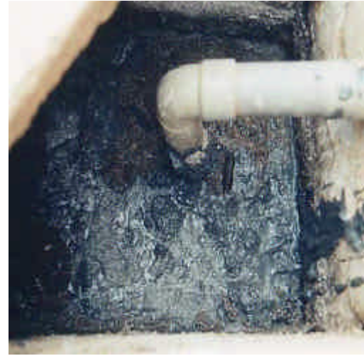
Figure 2-12: Top view of decanter with floating material
