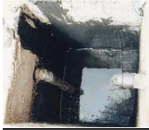
Figure 2-8: Top view into a decanter (outflow pipe on the left is partly missing)
