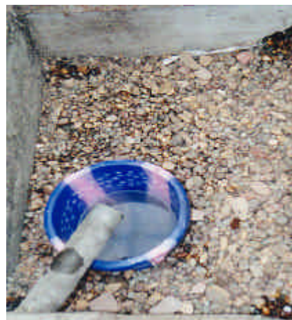
Figure 3-7: Photo of gravel filter with decantation / filter bucket
