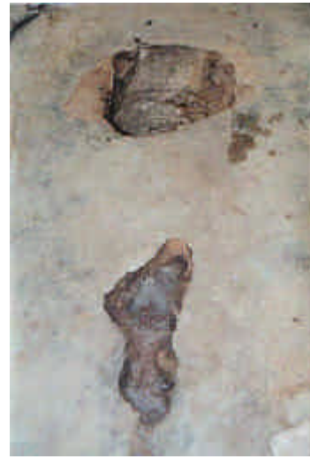
Figure 3-9: Local concrete corrosion
