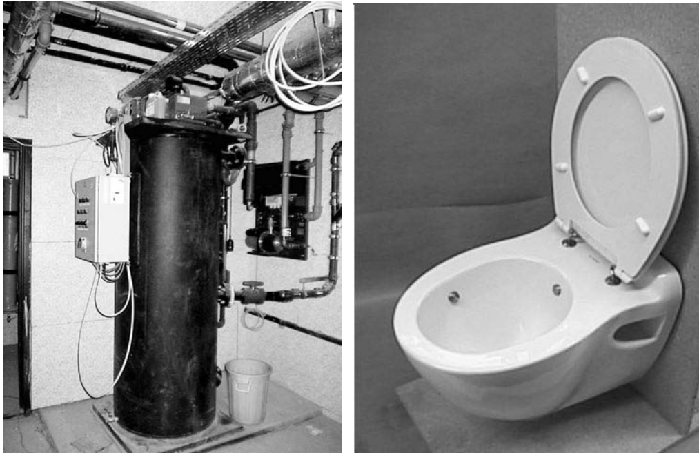
Fig. 4 Vacuum Pumping Station (Left) and Vacuum-Toilet of the Model-House
