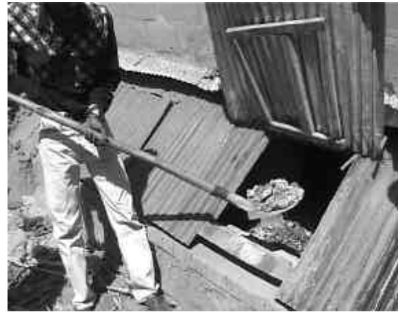
Figure 2: Emptying of a ecosan latrine
