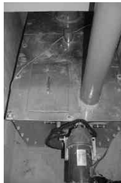
Figure 2: bio toilet treatment tank
