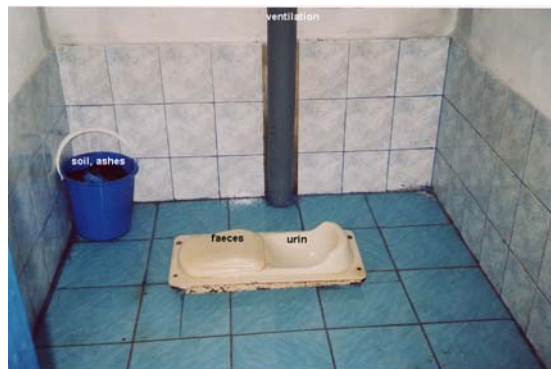
Figure 2. Interior of the u. d. toilet (Design TUHH)
