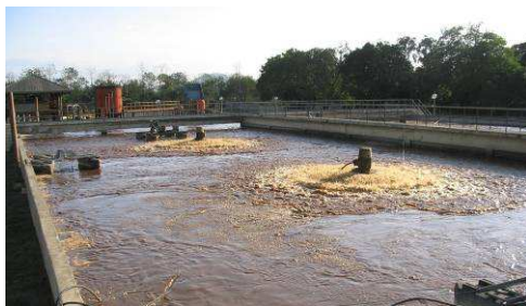
Activated Sludge Plant
