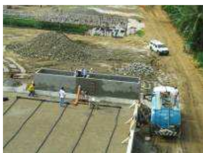
Header tank with distribution system
