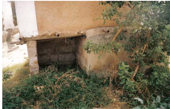
Figure 7. Convertible Overhang Latrine.
