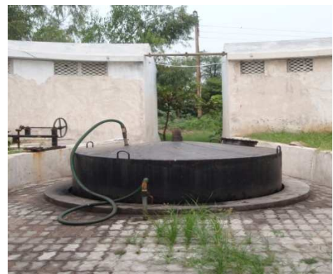
Fig. 13: The biogas plant inside the sanitation complex (source: Annik Staub, Sept. 2008).
