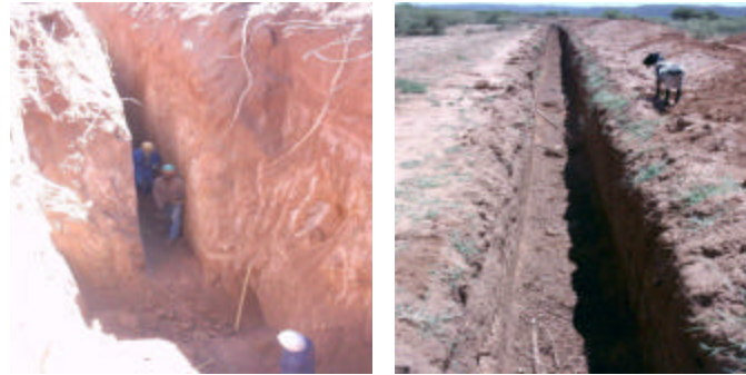
Example of excavation depths for both gravity (left) and vacuum systems (right) in Shoshong.
