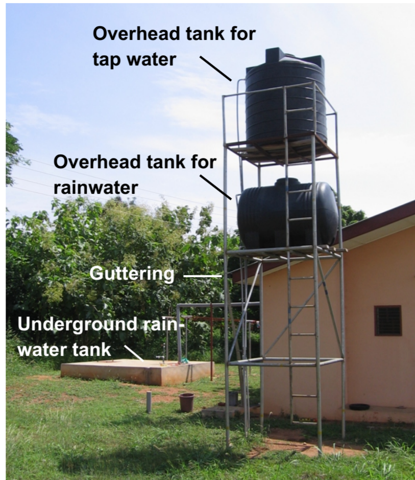
Rainwater harvesting (Bungalow at VVU campus)
