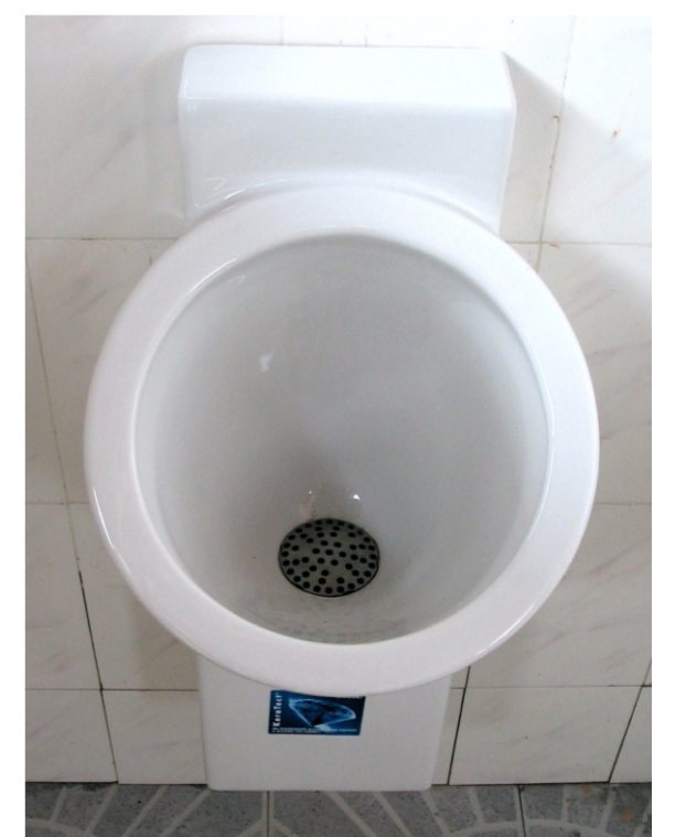
Dry toilet (Sanitary block, VVU campus)
