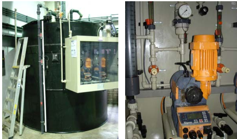
Figure 3-3 PAC dosing tank and pumps
