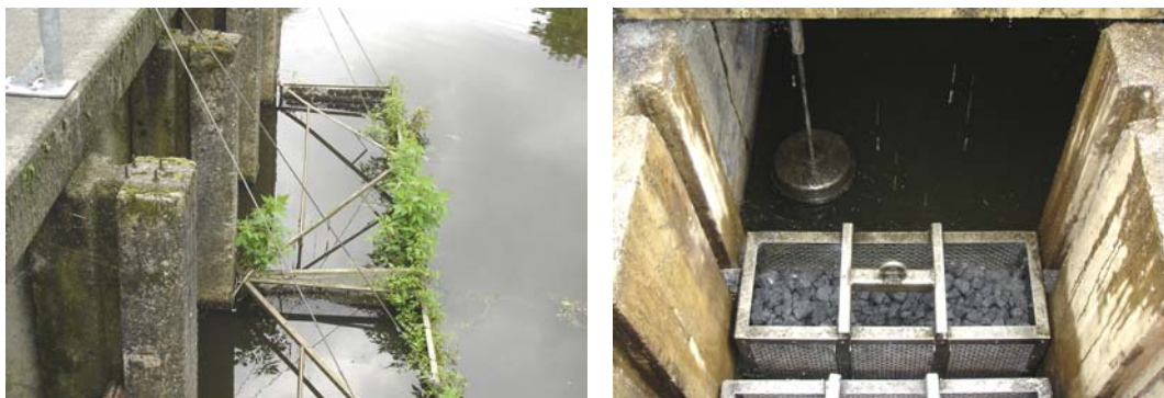
Figure 3-2 Water intake and rough filter
