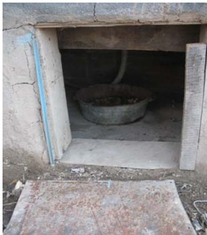
Figure 2: Single vault UDDT with too small container
