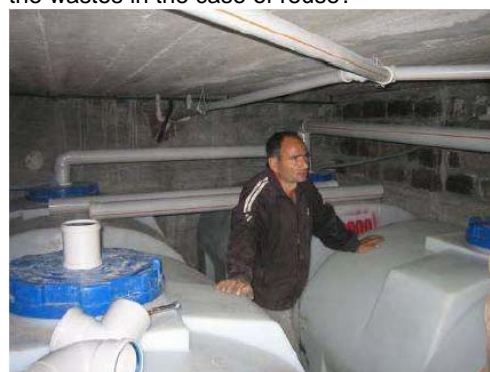
Figure 2 Urine tank in the basement of school, Armenia. Source: AWHHE in Samwel et al, 2007
