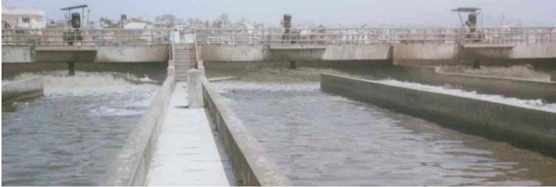
Picture 10. Sewer treatment plant of BASP, just upstream Pashupati temple.
