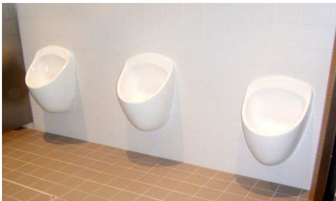
Fig. 6: Waterless urinals for boys from the Austrian company Hellbrok in the school building – hung lower than for adults (source: OtterWasser GmbH).
