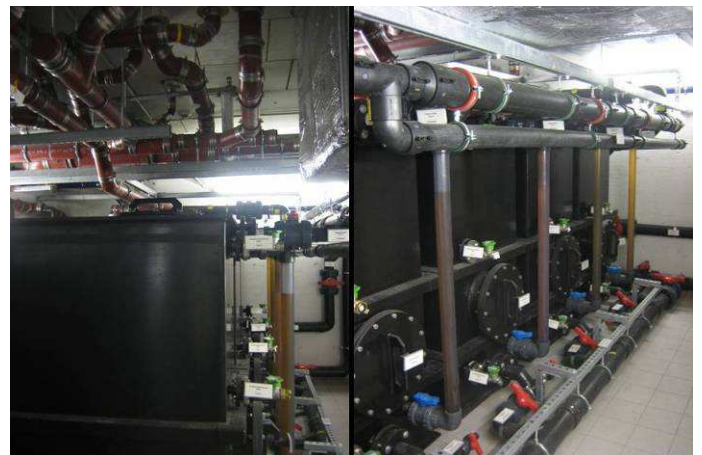
Fig. 5: Left: Plastic urine storage tanks in the basement of House 1 with connected urine pipework. Right: urine tanks with level indicating plastic pipes (source: L. Ulrich, April 2009).
