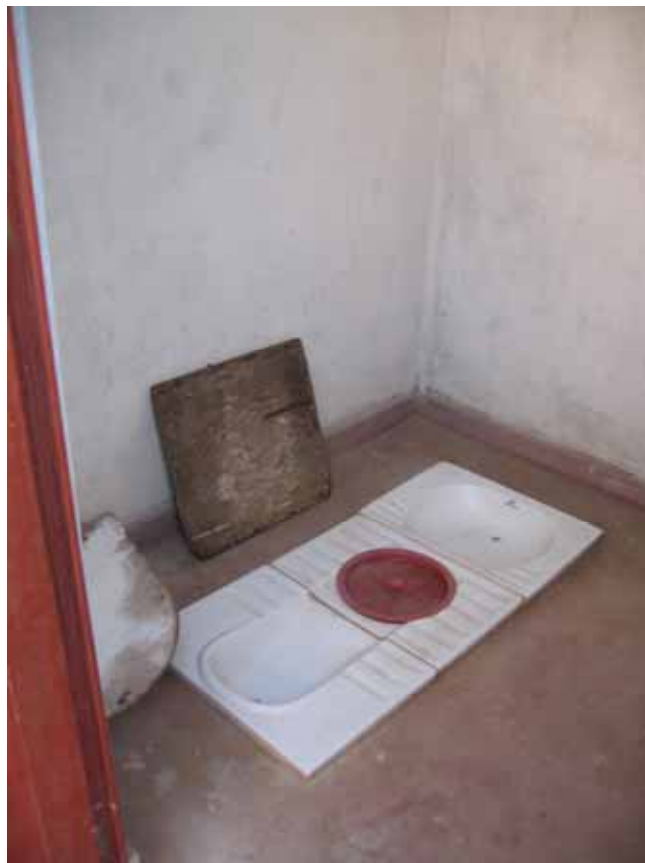
Squatting pan produced by Shital cermics in a toilet in Gujerat (photo ESF)
